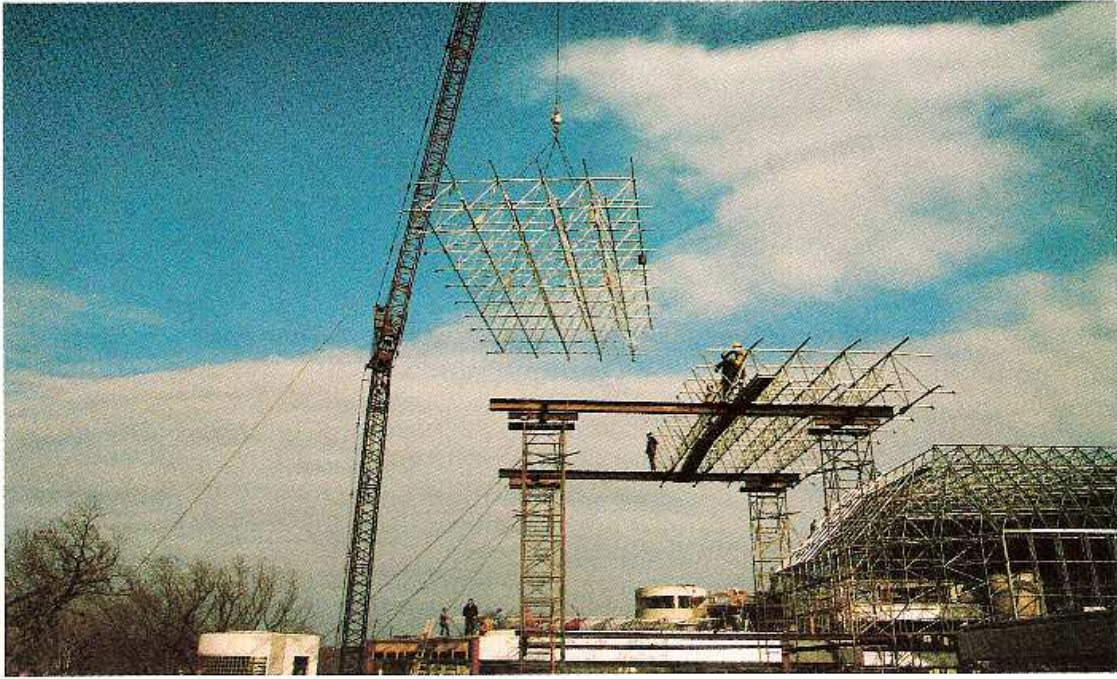
INTELSAT HEADQUARTERS BUILDING, WASHINGTON D.C. Erected by R.E. Linder Steel Erection Company, Inc.
